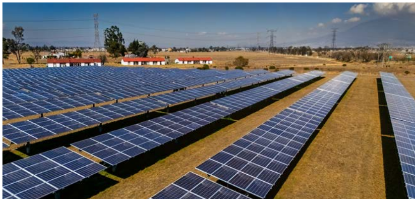
Renewable energy infrastructure in Mexico presents opportunities for investments toward electrification and grid modernization across North America, such as these solar panels in Michoacan, Mexico.
